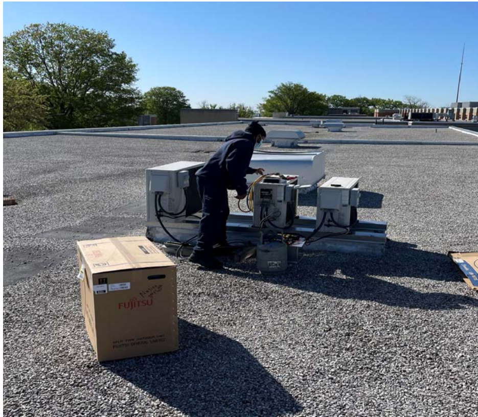
BEFORE – OLD UNITS
